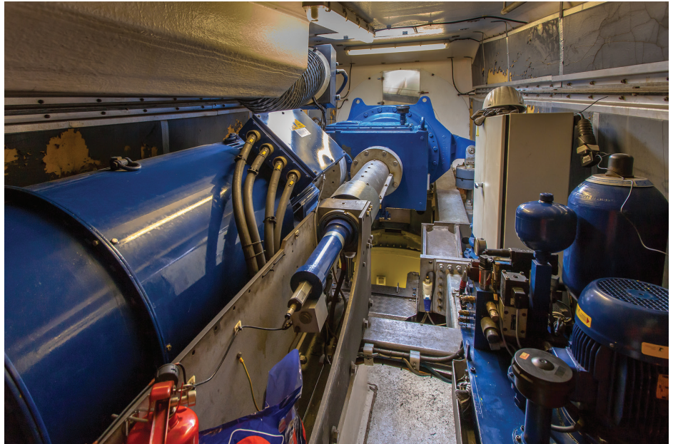
The wear generated in a wind-turbine gearbox is a function of load, speed, and lubricant condition. (Courtesy: Spectro Scientific, Inc.)
